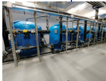
Multimedia filtration system
